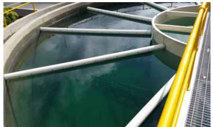
View from the top of the clarifier at the Yarwun Water Treatment Plant.
