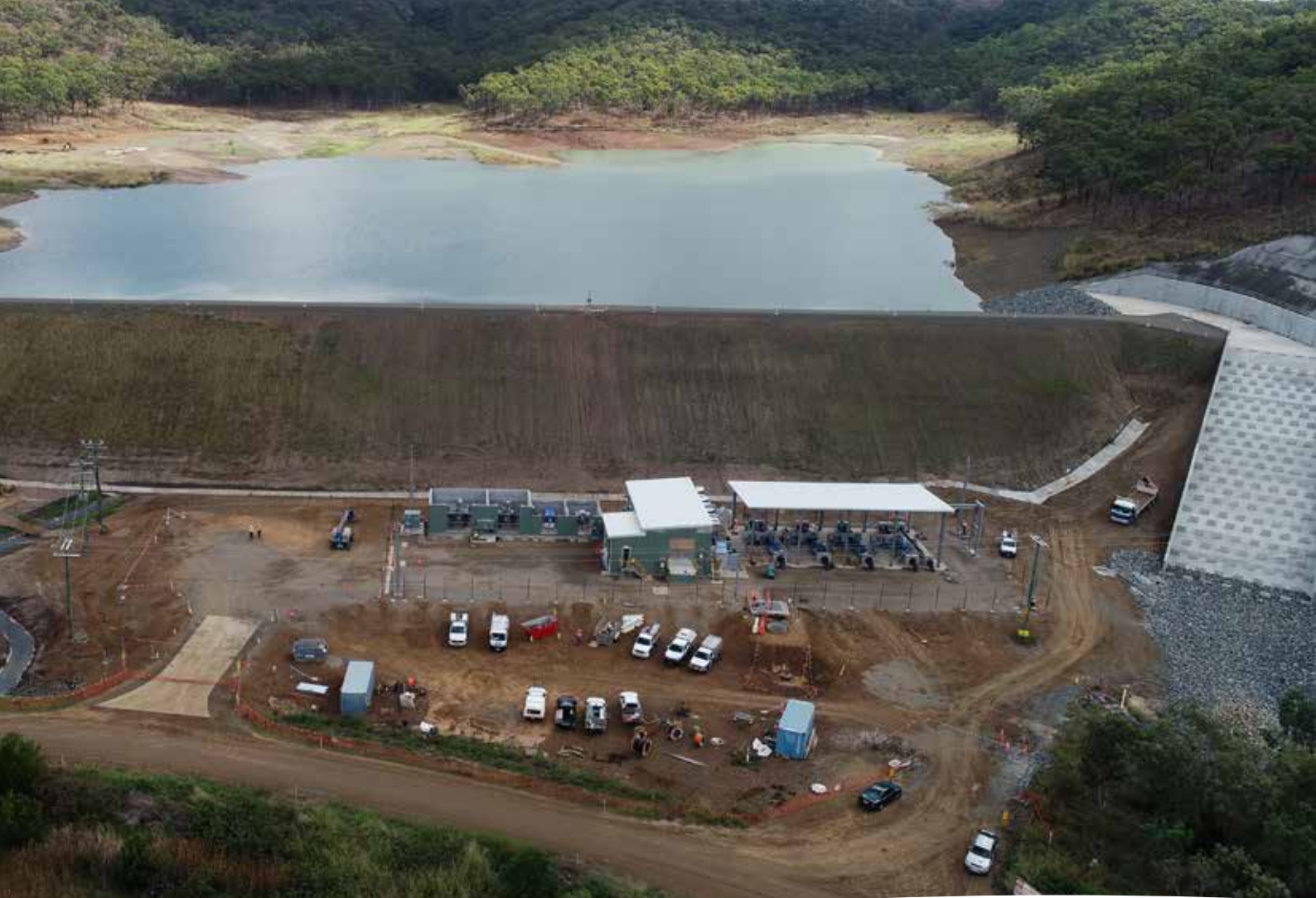
Progress of the construction of the Offline Water Storage Facility as at July 2018
